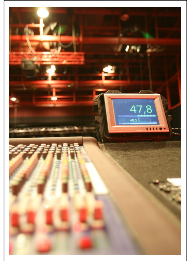
Figure 2: Mixing console with sound measurement device
