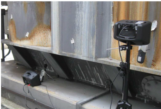
4.1. Speakers at short distance from transformer
