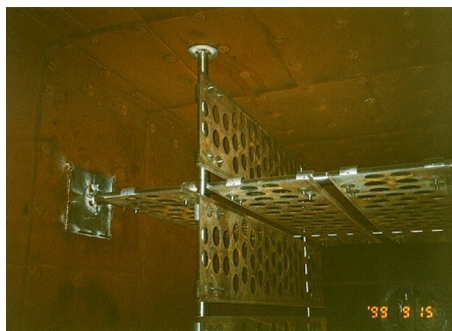
Figure 9: Baffle plate inside the duct.
