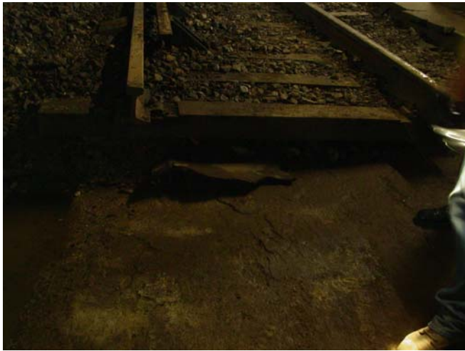
Figure 3: Cross section of the trackwork showing the larger than usual ties thinned on one side.
