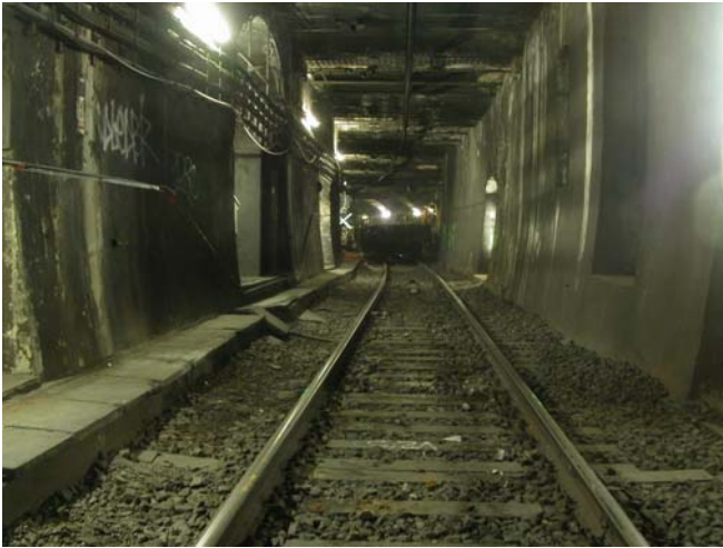
Figure 1: The tunnel before rehabilitation; note the reduced loading gauge and the structural connections of the track to the tunnel walls.
