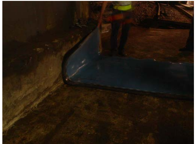
Figure 4: The resilient mat by Sylomer glued to the floor and lower walls of the tunnel.
