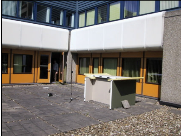
Fig. 6 Sound enclosure quench pipe.
