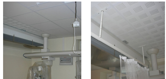
Image 4. The picture on the left shows the ceiling in the initial phase. The picture on the right shows the ceiling surface after reconstruction. The reconstruction meant that the existing ceiling panels had to be replaced to as great an extent as possible with panels with a higher absorption performance.
