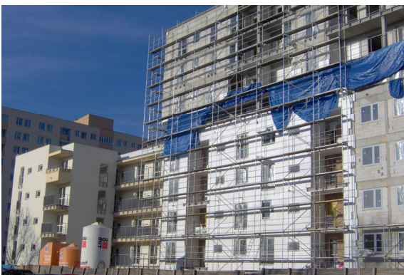
Fig. 1 ETICS applied to an old residential building constructed in 1910 and the same system used for a new building under construction in 2008.
