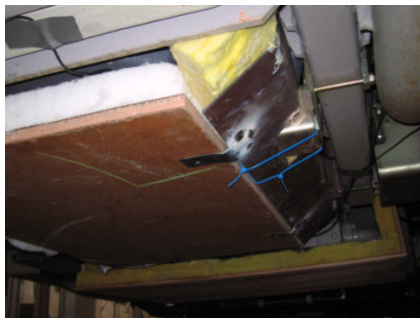
Fig.5 complete encapsulation of the Diesel engine.
