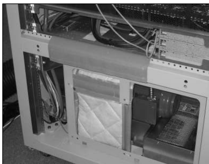
Figure 5. Electrical motor within housing and treatment.
