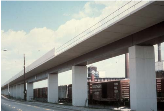
Fig. 9 MARTA Composite Steel/Concrete Aerial Structure at a Transition from Undamped to Damped With Sound Barrier Wall
