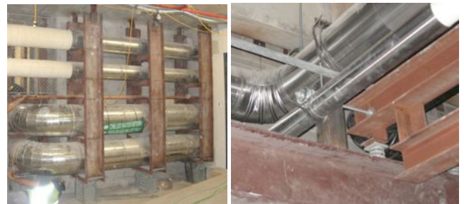
Fig. 6. Vibration Isolated Pipe Racks.
