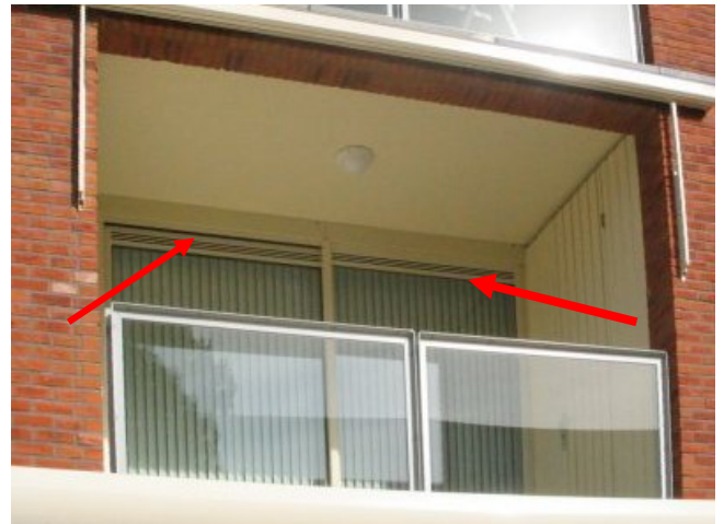
Fig 3 Ventilation grate near a ceiling outside
