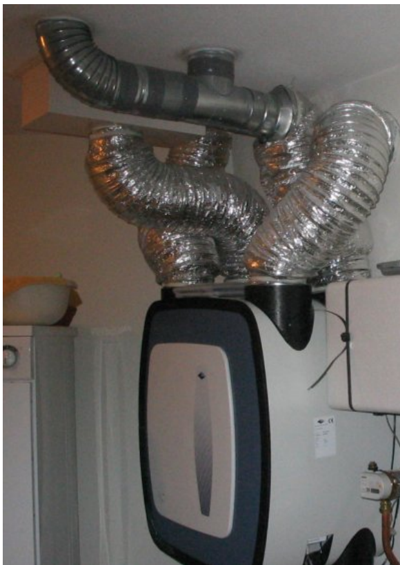
Fig. 2 Balanced ventilation unit with too short acoustical ducts and also with bends with too much resistance, which result in too much noise. L_{IA} varies from 34 to 52 dB.
