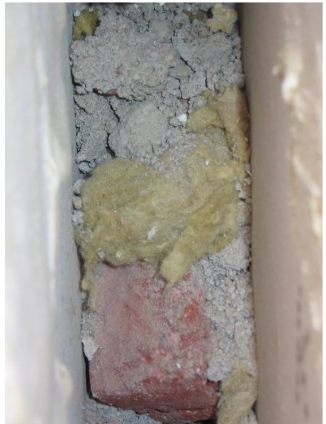
Fig. 4 The cavity of a cavity wall is near the ground floor no more a cavity. By cleaning the cavity the airborne sound insulation was improved from R_A = 46 to 59 dB.
