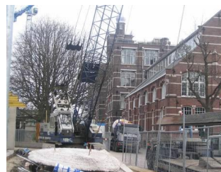
Figure 1a: Construction machinery in an inner city area with nearby newly developed apartments
