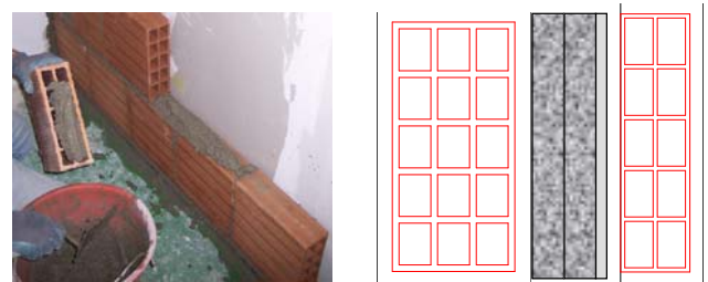
Fig.7 The hollow brick for the second masonry of wall B (left) and the whole wall (right).
