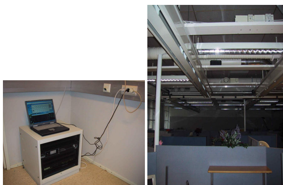
Fig. 4. Sound masking central unit and one of the black loudspeakers installed above electric shelf.
