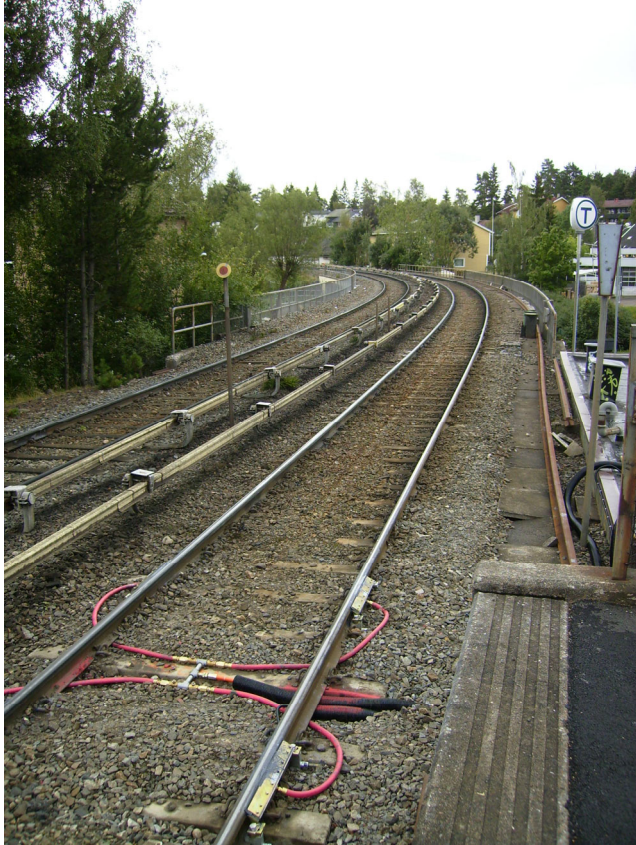
Fig.5 Lubrication system and the curve which has led to noise problems.
