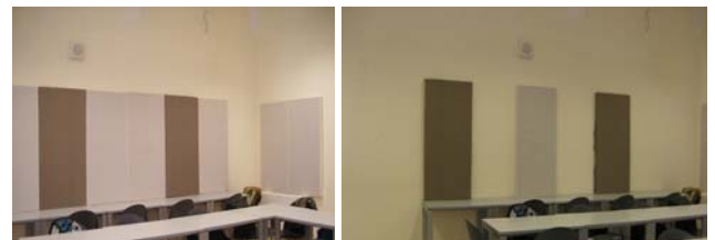
Fig. 8 Classroom T1 with insertion of absorbing boards.
