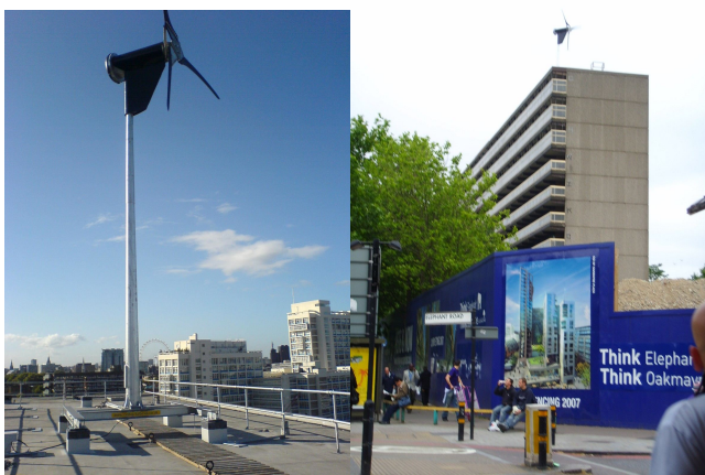
Fig 2.Proven 6 kW wind turbine on Ashenden House. Note the H-Frame mounting and the four concrete stubs
