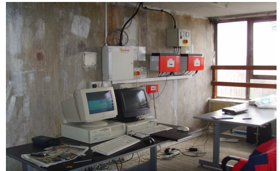
Fig 4.Flat directly beneath the turbine -electricity metering
